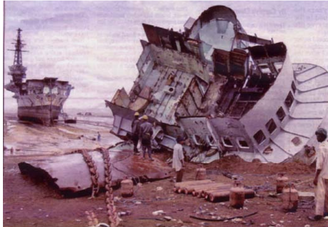
The Bridge & fore-part of the Island, part of the flight deck and cable deck have been removed
